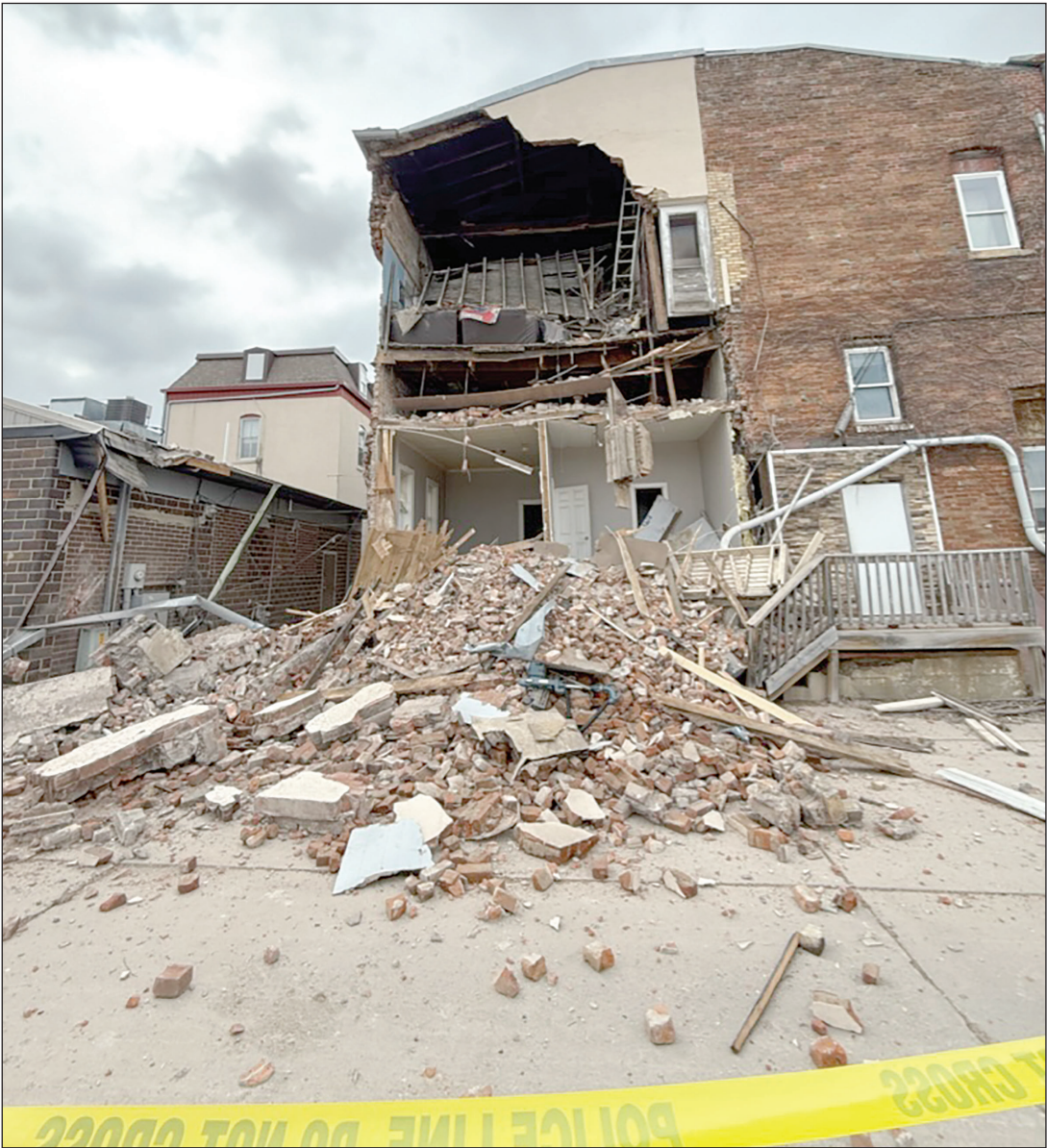
The back wall of the building at 115 South State Street in Waseca fell in two sections at about 1:15 the afternoon of Wednesday, April 2. No one was injured; tenants have been helped in finding temporary housing. Pioneer photo by Eli Lutgens
