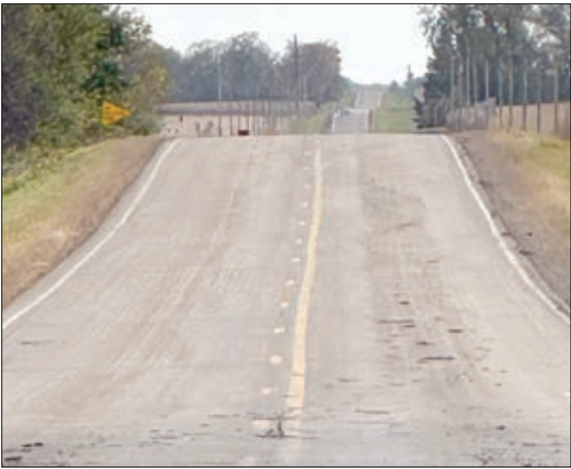
VISUAL TRAP - This roadway in Waseca County provides an example of a "visual trap." An unfamiliar driver could easily believe this road continues straight ahead, but the hill is concealing a curve. Pioneer photo by Deb Bently
